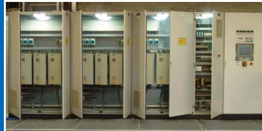
In-house engineered state-of-the-art controls
